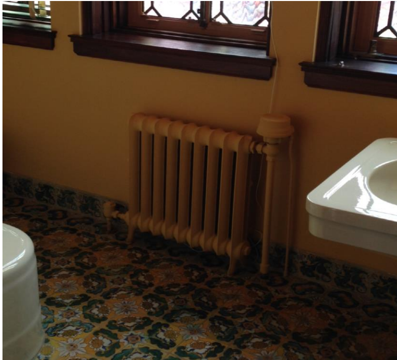
Radiator in the Fourth Floor Bathroom Photo credit: Kristy Cambron on YouTube
