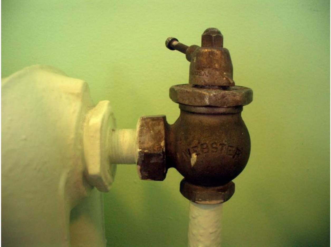
Close up of the radiator in the Kitchen of Ca' d'Zan
